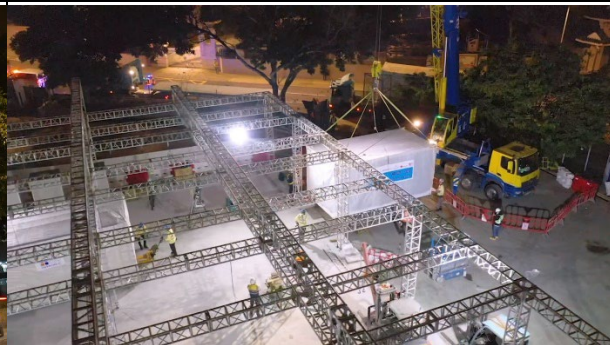
Modular Integrated Construction (MiC) approach was adopted for swift delivery of the vaccination centre.
