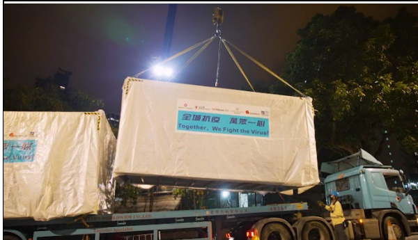
Modular units were prefabricated in a factory in mainland China, with production and delivery to Hong Kong taking only seven days.
